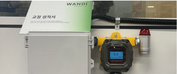
Gas Detection System Status Board
