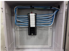
Inspect the Operating Status of SPDs
