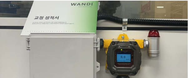
Gas Detection System Status Board
